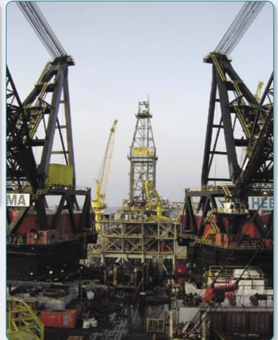
The completed TLP with the Thialf and its giant cranes in the foreground
