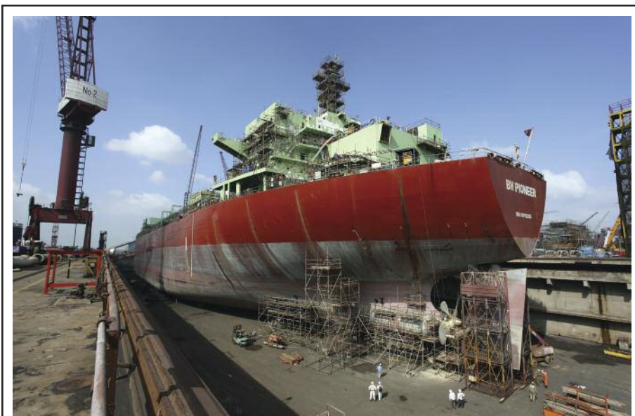
Production is scheduled to commence at the Cascade and Chinook Lower Tertiary fields in mid-2010 using the Gulf’s first floating production, storage and offloading system. When commissioned in more than 8,500 feet of water at Walker Ridge 249, the BW Pioneer will establish a world water depth record for an FPSO installation. The FPSO is shown here undergoing refurbishment and conversion work in Singapore.
